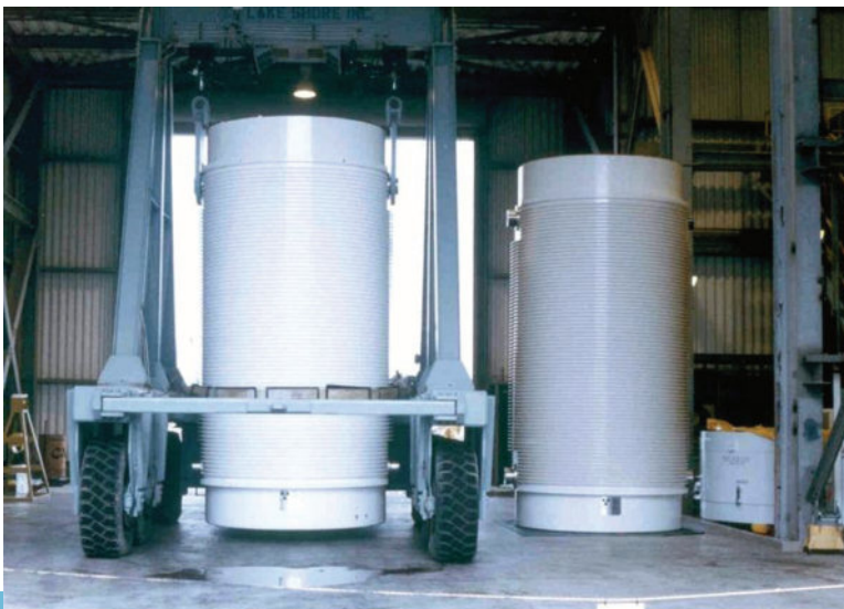
FIGURE 4.29 Dry storage of spent fuel.
