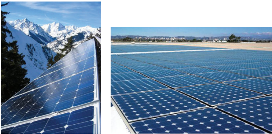
FIGURE 6.37 High power PV systems. (Images are courtesy of the US Department of Energy, Washington, DC.)
