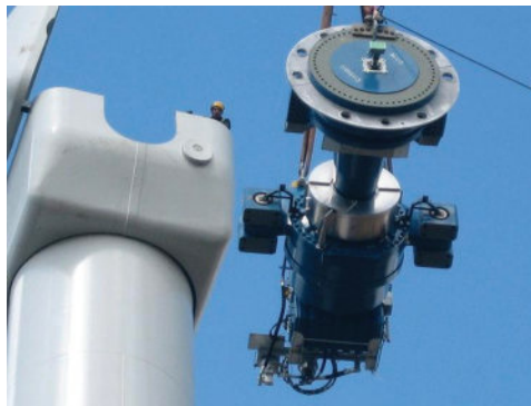
FIGURE 6.58 Lifting of gearbox and brakes of HAWT. (Courtesy of Paul Anderson through Wikipedia.)
