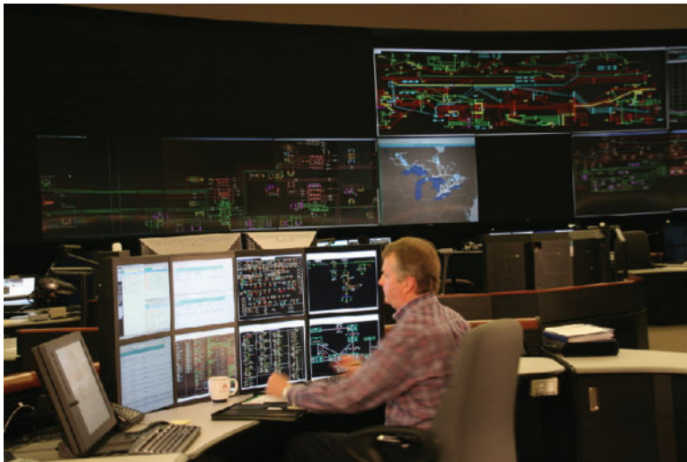
FIGURE 2.29 Control center. (Image courtesy of Alstom Grid, Redmond, Washington.)
