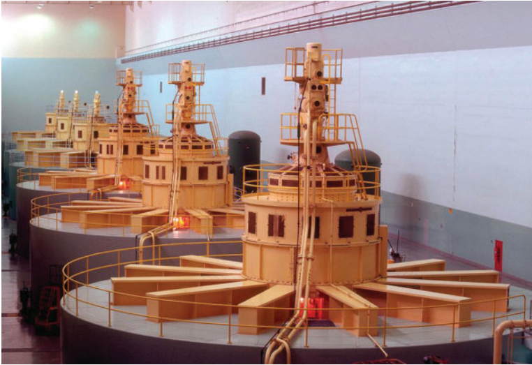
FIGURE 4.5 Hydroelectric turbine-generator units at the lower granite power plant, Walla Walla, Washington. (Image courtesy of U.S. Army Corps of Engineers, Louisville, KY.)
